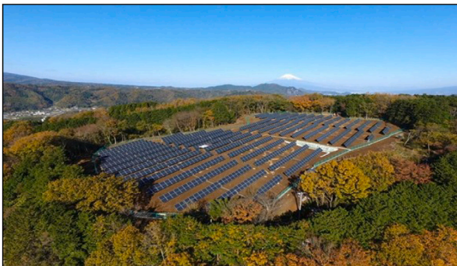
Fig. 3. A PMGD installation located on the outskirts of an urban area in Chile.
